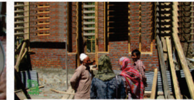
Construction of one of the 20 houses that were fully reconstructed by AMAN for the survivors of 2014 floods.
