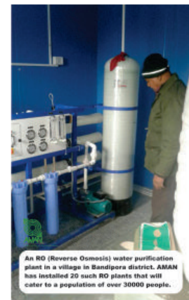
An RO (Reverse Osmosis) water purification plant in a village in Bandipora district. AMAN has installed 20 such RO plants that will cater to a population of over 30000 people.
